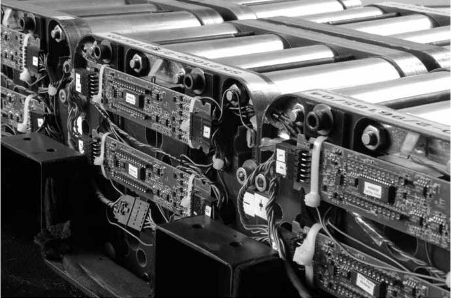
Figure 3.1 Typical large-format lithium-ion battery system.
