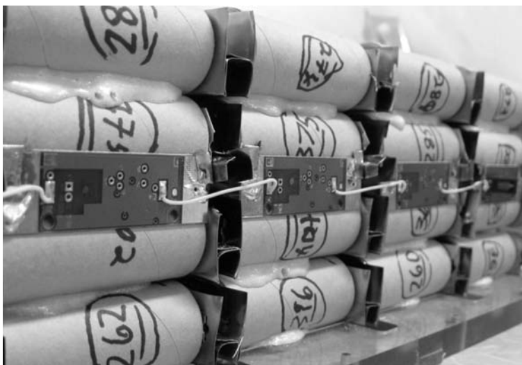
Figure 5.86 Cell boards mounted directly on small cylindrical cells.
