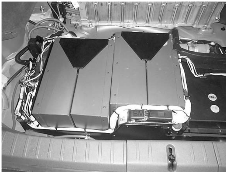
Figure 5.85 Spaghetti in a centralized traction pack for a Prius PHEV conversion. Note the wire harness (with 80 or so white wires) routed from the BMS (bottom) to the various batteries.
