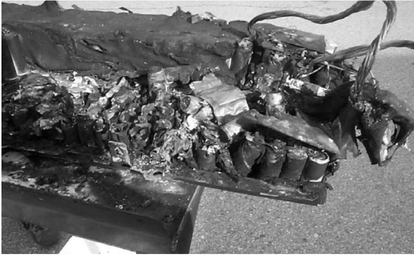
Figure 1.4 The same battery from Figure 1.3, after the fire.
